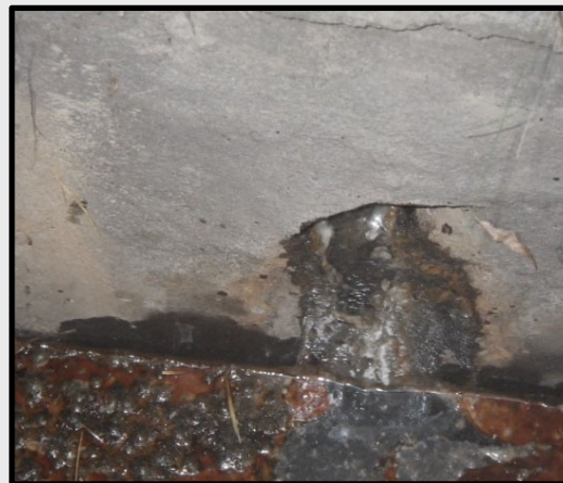
Sanitary sewage may be present if there is black staining inside the drainage pipe; visible evidence of sanitary waste (such as toilet paper); or opaque or gray water. Sewage may originate from septic tank overflow pipes or improperly disposed waste from travel trailers
